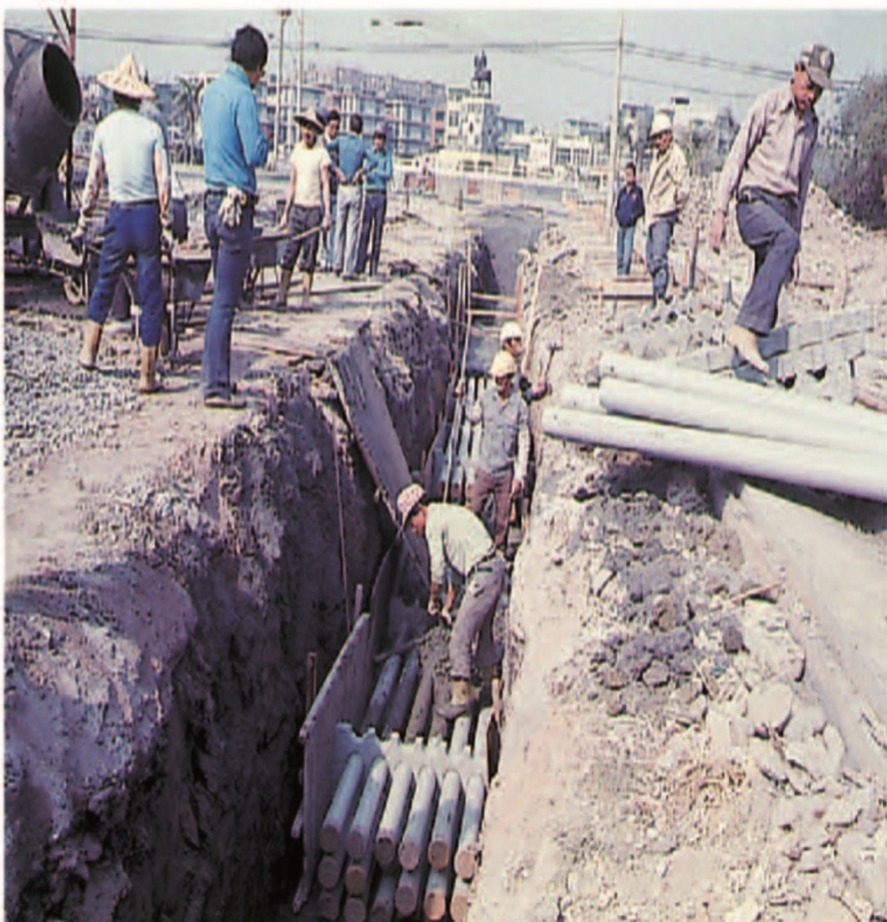
▲电气工程 Electrical engineering
